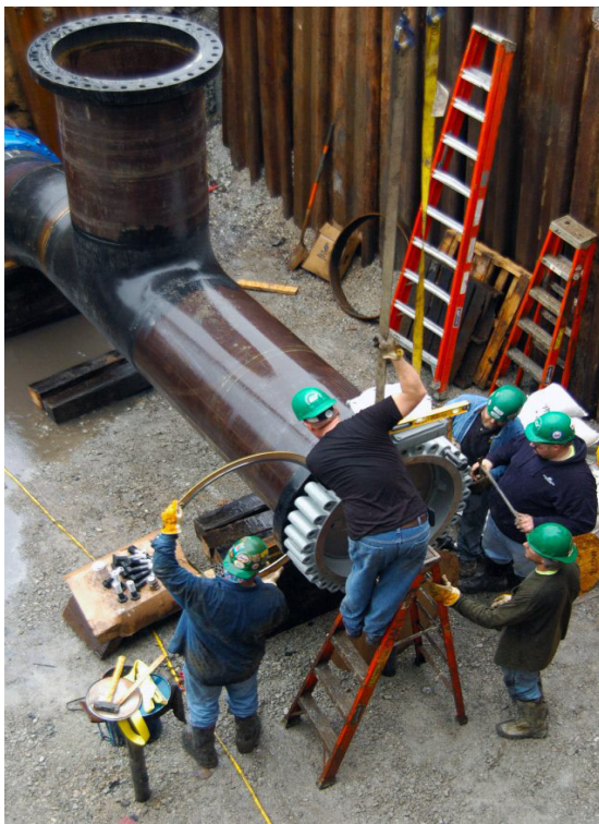
Waldinger Corporation employees fit a graphite seal (circle held by worker on the left) between a chilled water pipe and a new valve outside the City Campus utility plant.
