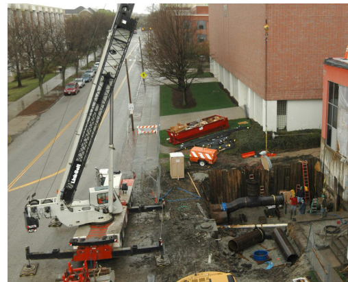
A crane lifts a valve into place outside UNL's City Campus utility plant.
