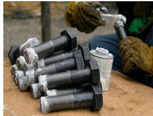
A worker applies anti-seize lubricant to bolts used to attach a 36-inch valve onto new pipes leading into UNL's City Campus utility plant.
